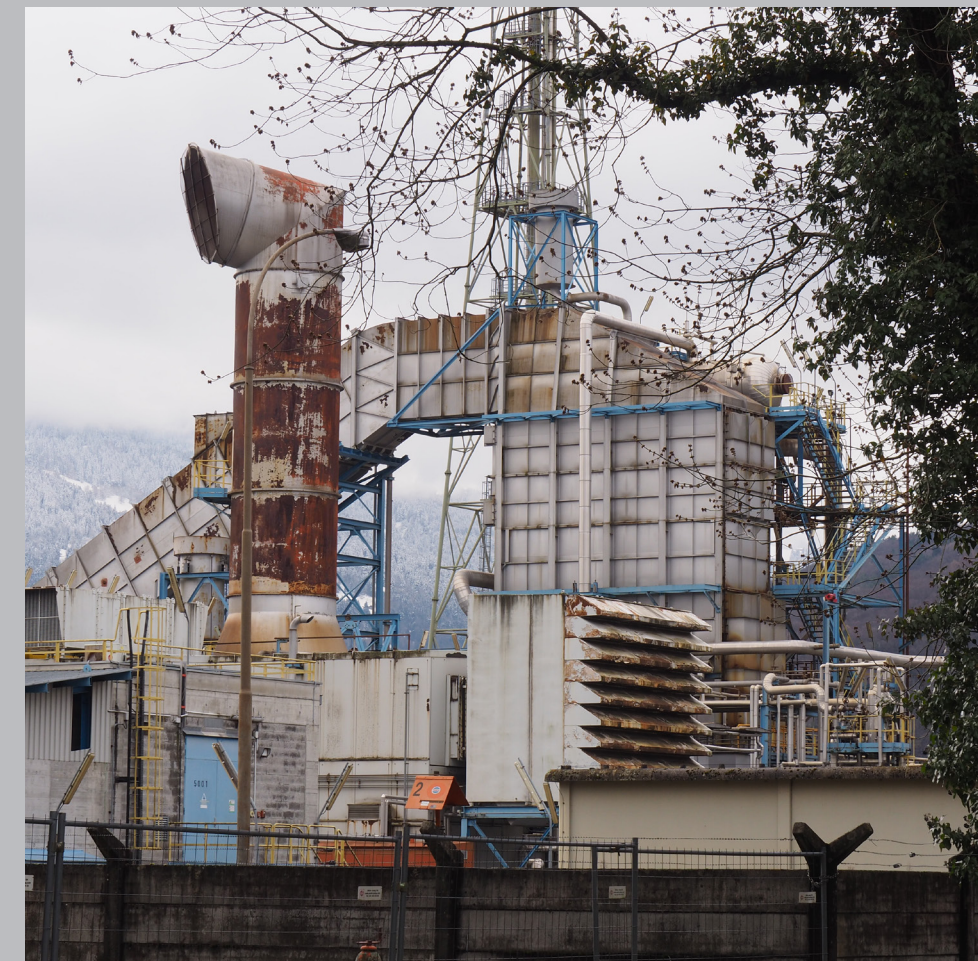
ventilation: metallic plates of various sizes
