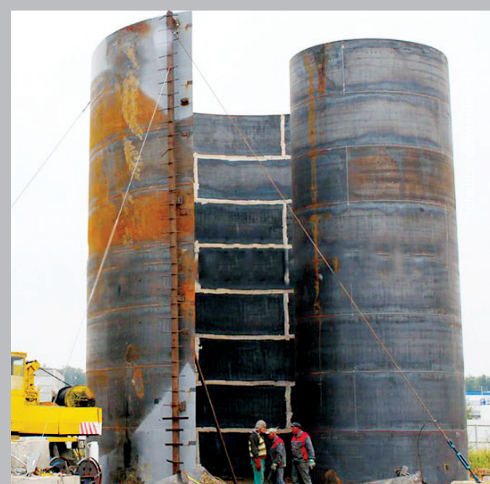
coiling method: welded in factory, up to 16m long, weight adjusted for transportation, unrolled on site
