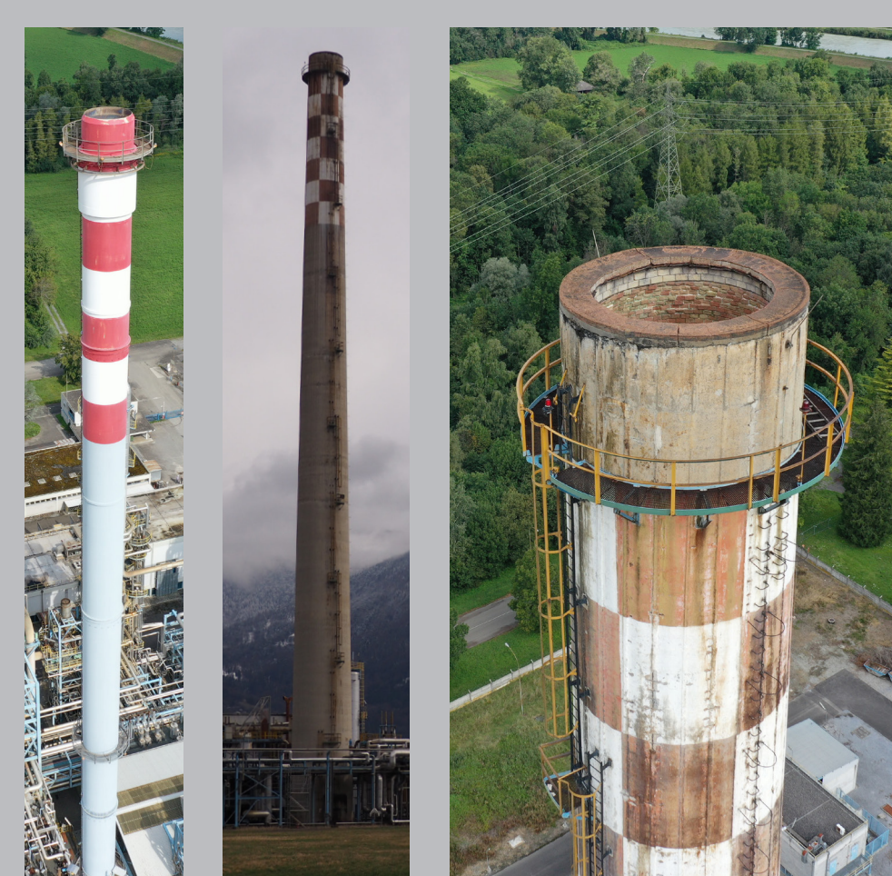
chimneys : 2x bricks 100m + 1 x steel + steel torch ("without smoke")
