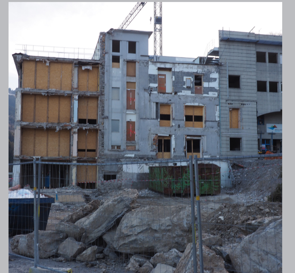
deconstruction of the east wing of Monthey hospital, providing reused insulation and concrete
